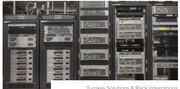
Turnkey Solutions & Rack Integrations
